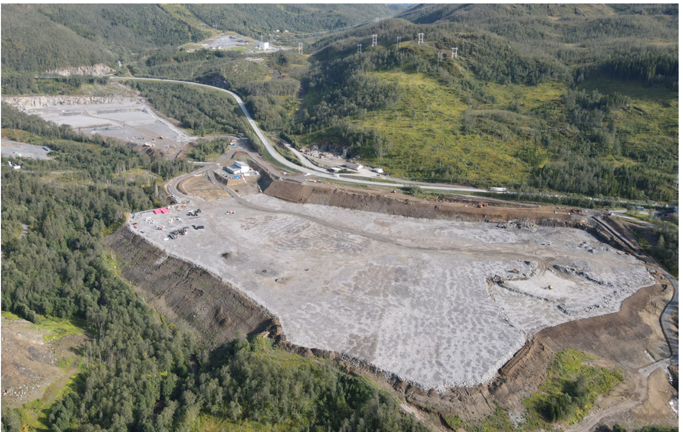
Narvik Green Ammonia site in Kvandal, close to Narvik – where the initial ground works and substation are now complete
